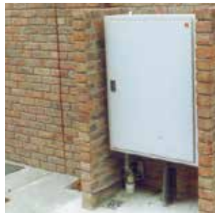
Six meter cabinet
