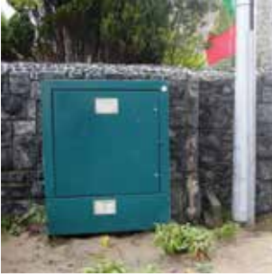
District Regulating Installation (DRI)
